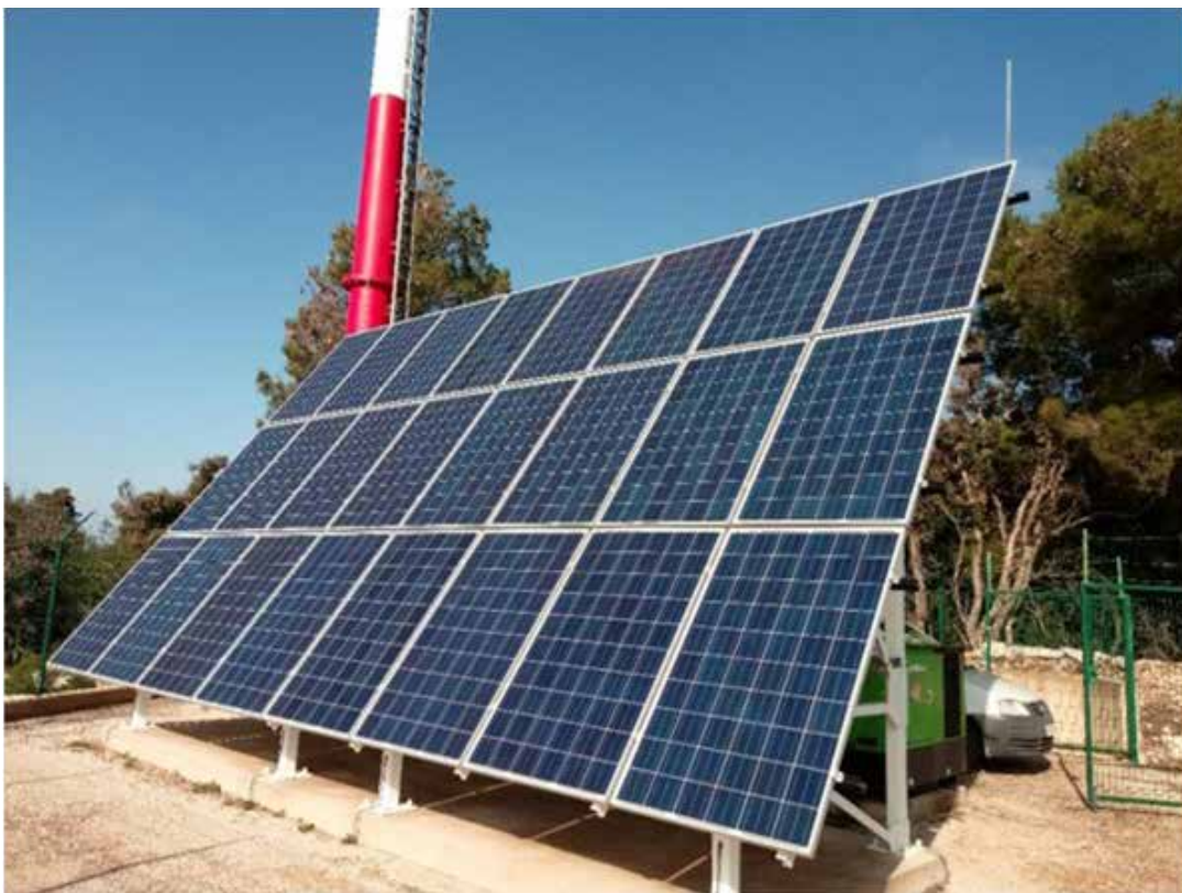
Figure 5: Ground-based navigation facility (DME - Distance Measuring Equipment) on Lošinj Island, Croatia, powered primarily by solar energy (Photo courtesy of Croatia Control).
